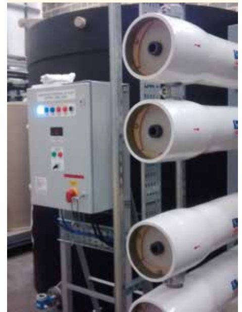
The secondary Reverse Osmosis Water Plant.
